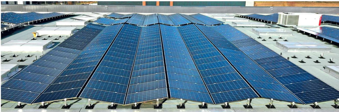
Example of a roof equipped with a photovoltaic plant
